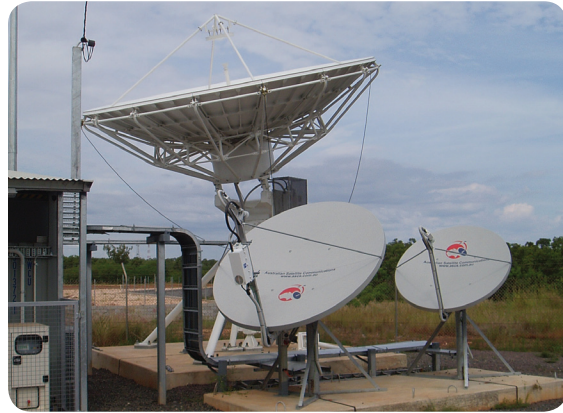
ASC installed teleport infrastructure in Darwin
