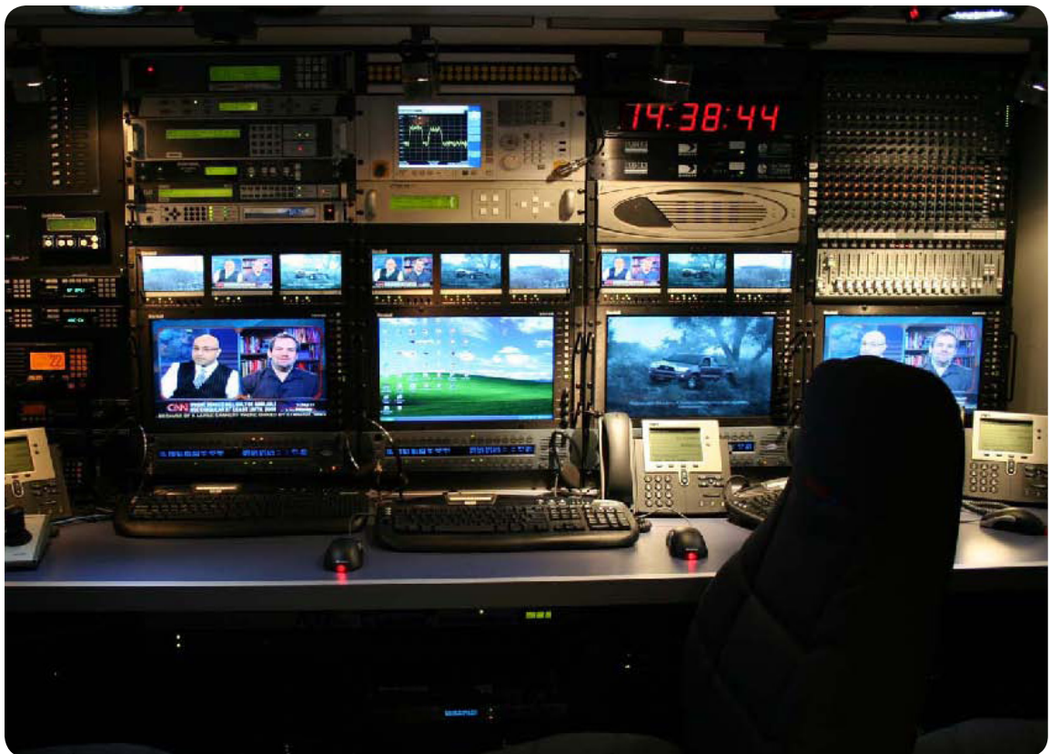
Main Technical Work Area — Unified Command Vehicle
